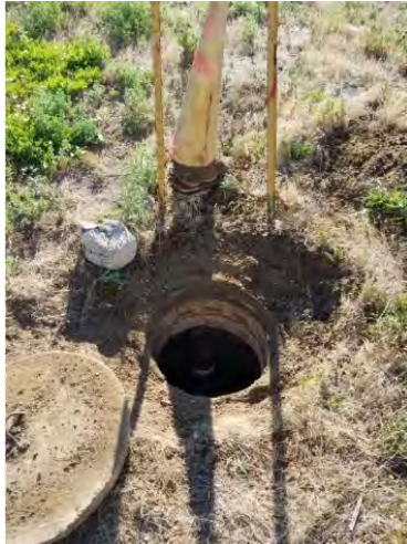
Image 2 – OWTS 1 Septic Tank
